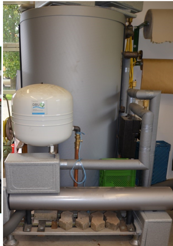
Heat storage and heat exchangers
